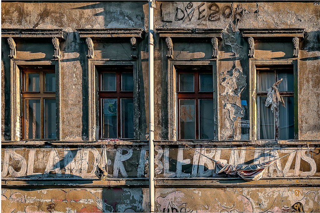
Broken [ID: B_MI_0197]
